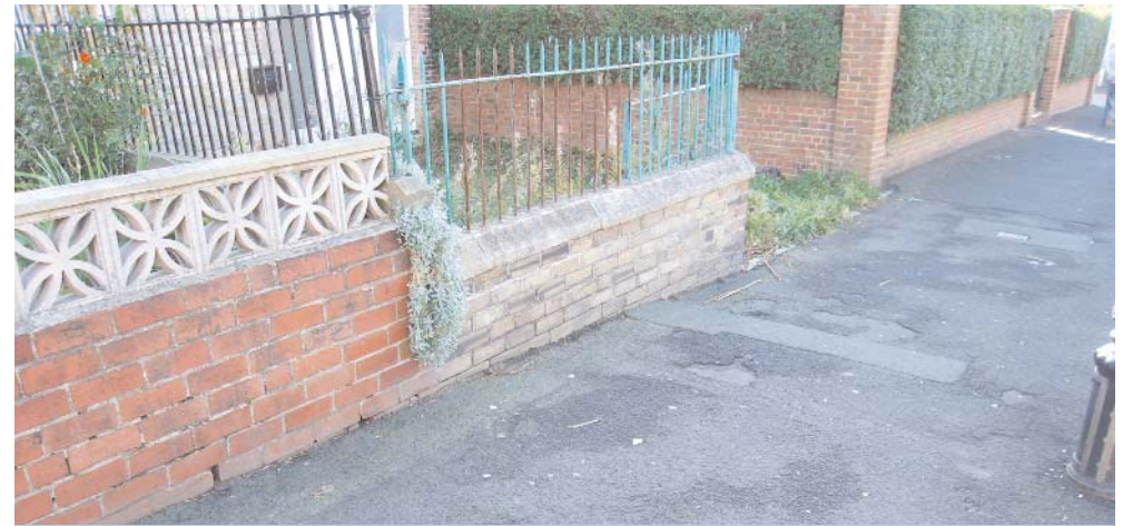
A mis-match of boundary walls and poor quality surface materials detract from the general streetscape and setting of historic buildings on the southside of Front Street.
