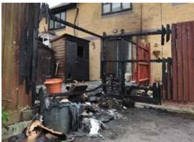
Damage caused by a wheelie bin fire
