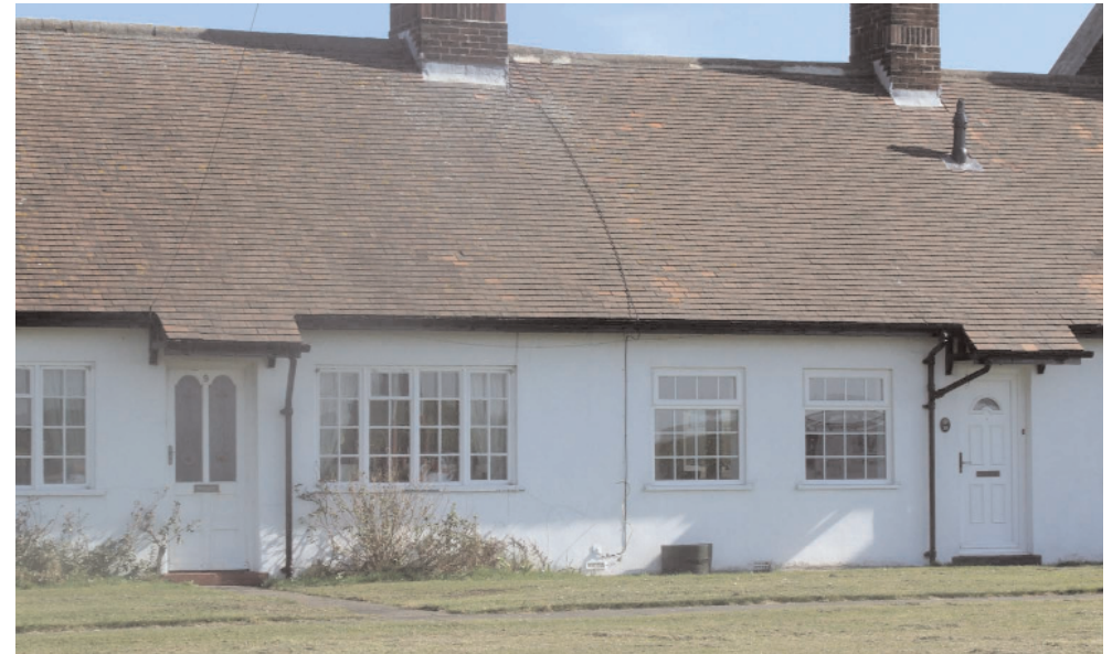
Changes to the window openings and windows to accommodate replacement PVC units have insensitively altered the historic form of the property to the right; the property to the left has retained its original appearance.
