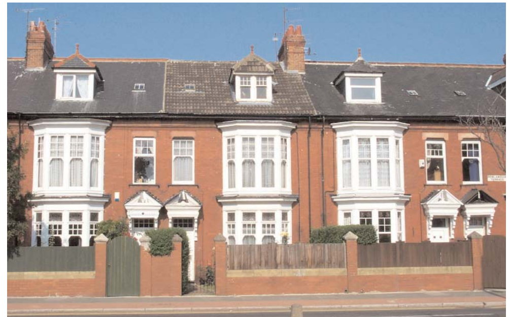
The impact of changing roof materials, (centre), and replacing original timber windows with uPVC (right) or diverting from a colour scheme (porch, far right), on otherwise uniform terraces is detrimental to the special character and appearance of an area.
