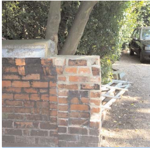
A gate pier missing its decorative capping stone
