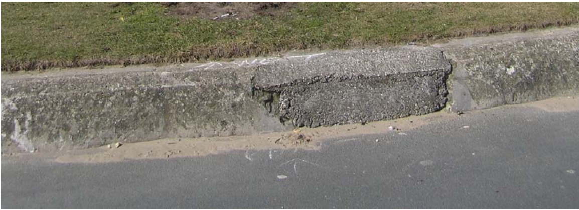
Photograph 1: Original damaged concrete edging
